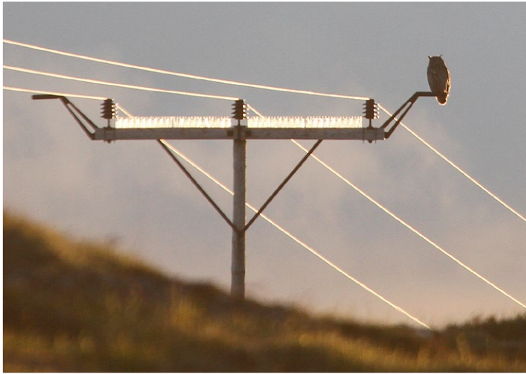
CEDREN has developed an elevated prolongation of the power-pole cross-arm, providing safe perching for eagle owls. Photo: Jan Ove Gjershaug
